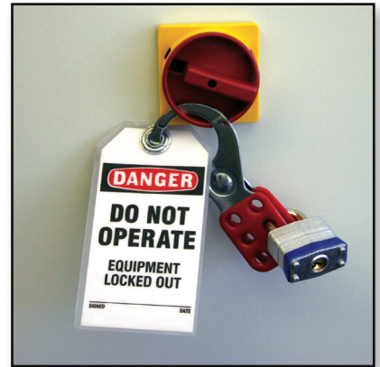
Locked out and tagged out (LOTO)
