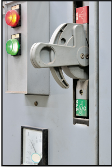
Main disconnect switch
